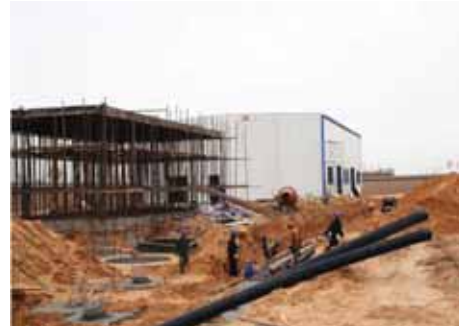
Compressed Air / Nitrogen Station
